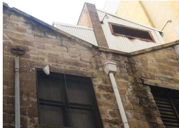
DETAIL OF STEPPED CRACKING SUGGESTING MOVEMENT ALONG THE ROOFLINE AND SPALLING TO PARAPET
