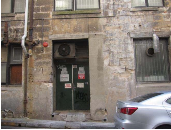
THE REAR ACCESS TO THE GALLIPOLI CLUB BAR (12) PARTIALLY INFILLS THE CENTRAL BAY.
