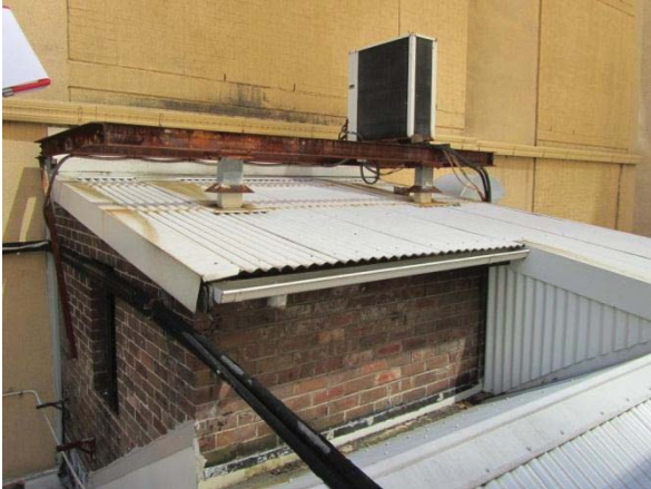
LIFT MOTOR ROOM
