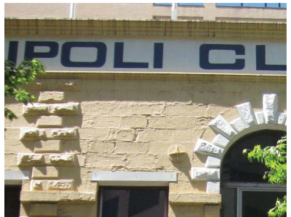
CRACKING TO THE PARAPET
