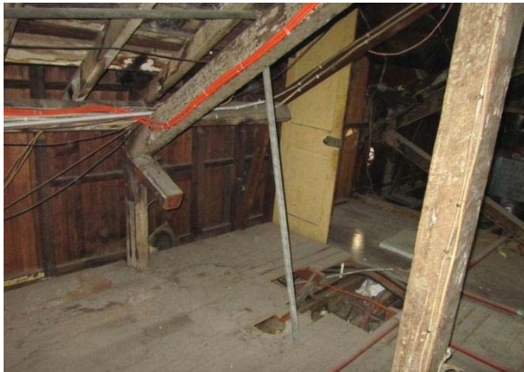
DETAIL OF ONE OF THE MISSING MEMBERS
