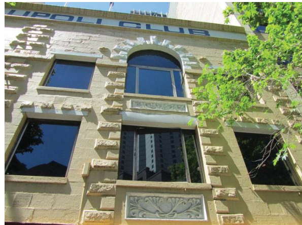
DETAIL OF THE FAÇADE OF NO. 14 SHOWING THE ALTERED WINDOWS AND C.1910 ART NOUVEAU SPANDRELS WITHIN THE INFILLED CENTRAL BAY
