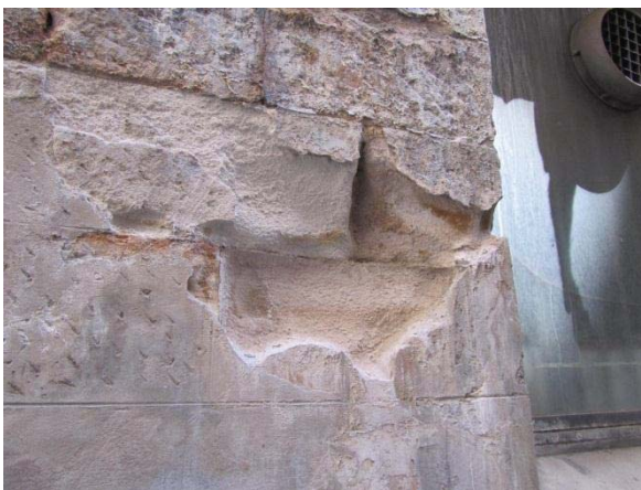
SEVERE SPALLING/ DELAMINATION OF STONE TO THE NORTHERN STORE (GROUND FLOOR)
