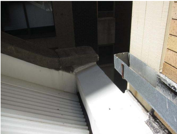
DETAIL OF BOX GUTTER, SOUTH WALL GUTTER AND DISCHARGE TO THE REAR LOFTUS LANE (SE CORNER)
