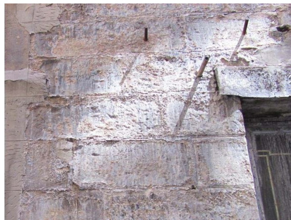
DETAIL OF SALT DAMP TO THE NORTHERN STORE
