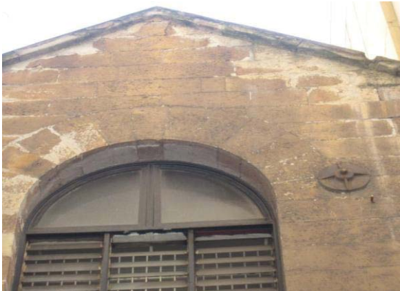
DETAIL OF THE GABLE END SHOWING DELAMINATED (SPALLING) STONE BENEATH THE PARAPET CAPPING
