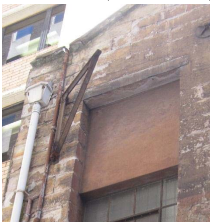
DETAIL OF THE REMNANT JIB HOIST AND INFILLED WINDOW (TO FIRE STAIR)
