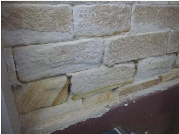
VIEW OF FRETTED AND DELAMINATED STONEWORK TO LEVEL 1
