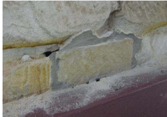
PATCH REPAIR WITH STONE VENEER ABOVE THE BUILT OUT BRICK WALL (LEVEL 1)
